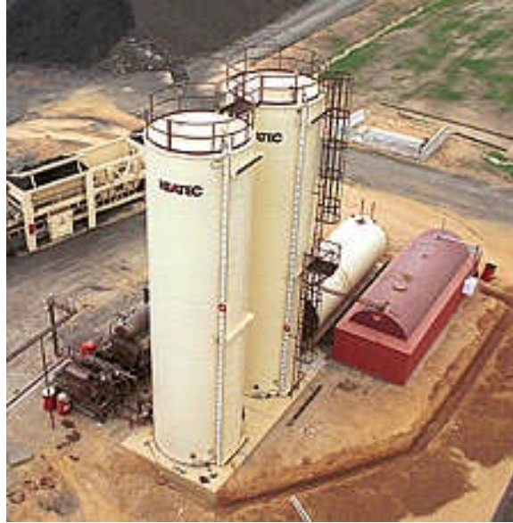
Figure 5: Vertical Asphalt Binder Storage Tanks (Courtesy Heatec, Inc.)
