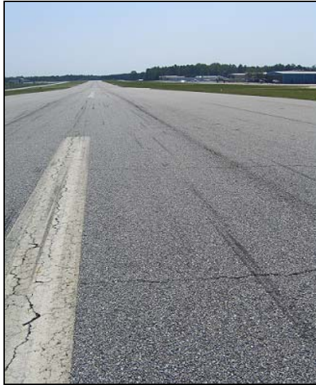
Figure B6 Transverse cracking along Runway 14-32 at Griffin-Spalding Airport
