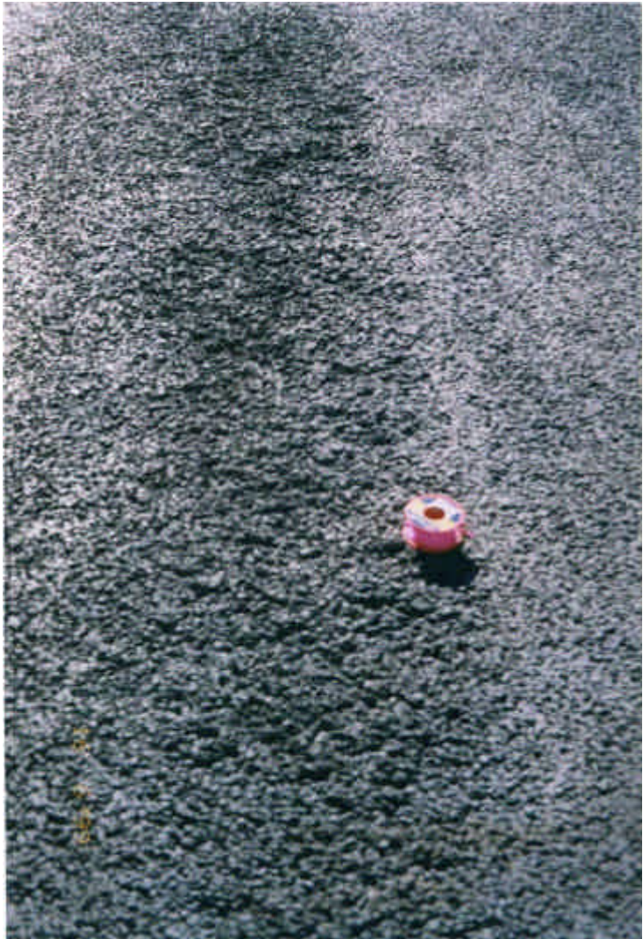
Photo 8 Typical open textured area caused by dragging of mix
